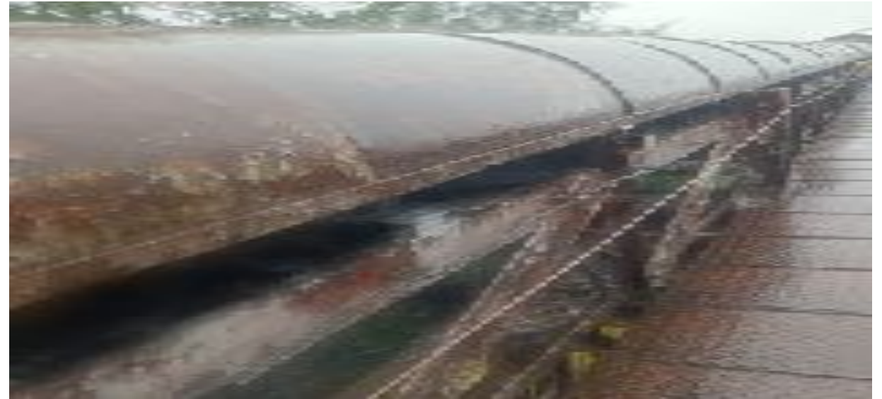
Rusted covers (Before)
